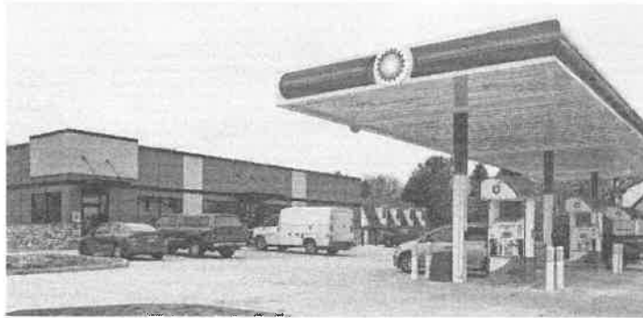
The new gas station complex constructed by Quasius Construction is pictured March 7, on North Rapids Road and Menasha Avenue in Manitowoc. It is also home to The Spices dine-in bar and restaurant at the site where Vogel Auto Body and John's Used Car Sales used to sit. GARY C. KLEN/USA TODAY NETWORK-WISCONSIN
